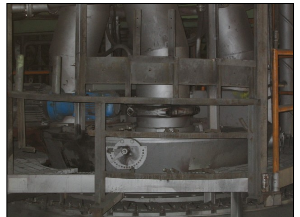
Classifier Outlet Pipes
